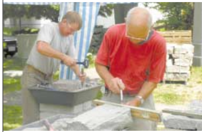
An open house was recently held at the Babcock Smith Museum in Westerly. United Builders Supply provided tools and stone from their "Westerly Pink" quarry for use in demonstrations. Bruce Brawlaey and Sai Capalbo, local stone masons from Westerly, demonstrated how to cut and dress granite using hand tools. A large piece of granite was split in half using "feathers and wedges." All work on the stones was done by hand, the only difference between 2010 and 1910 was the use of an electric drill to make the holes for the "feather and wedges."
