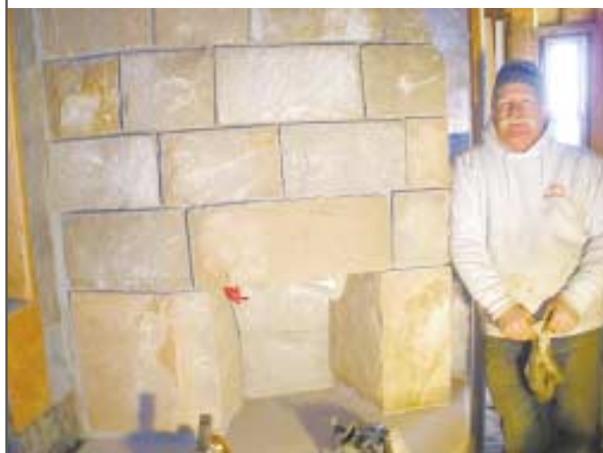
Local mason, Fred Lindsley, shows a hand-carved Westerly Pink fireplace. The firebox was carved from a single piece of Westerly Pink Granite. The Westerly Pink Veneer was provided with sawn tops and bottoms. Fred finished each block by hand. Materials were provided from the recently re-opened quarry owned by United Builders Supply.
