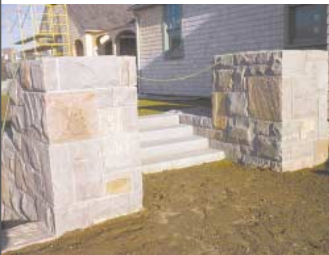
Westerly Pink Granite columns with Westerly Blue Granite steps at a home in Westerly. United Builders Supply provided the Westerly Pink blocks with the tops and bottoms sawn. Fred Lindsley, a local Mason, along with his crew, hand dressed each piece to form the columns.
