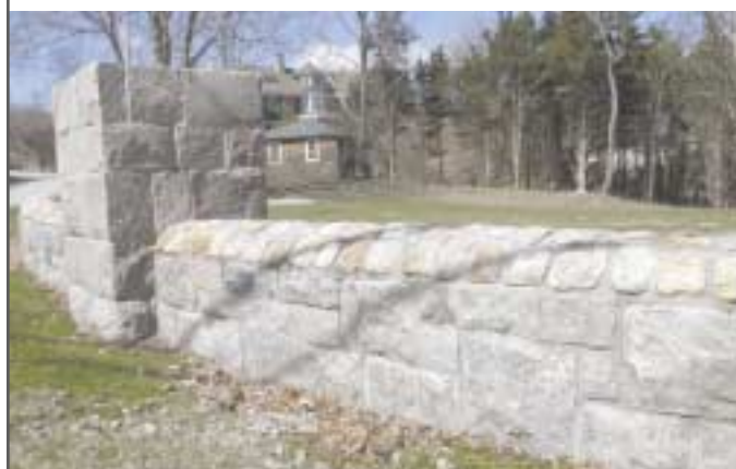
This picture shows the use of Westerly Pink in a recent restoration of a historic wall in Watch Hill. Westerly Pink was integrated with existing stones on the site to restore the wall to its' original splendor.
